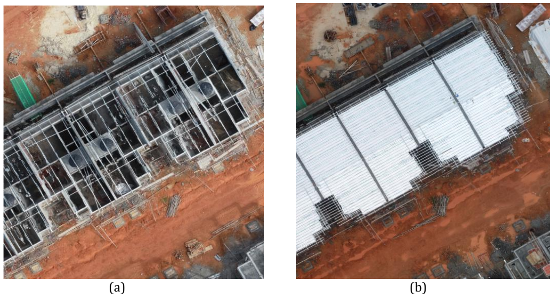
Figure 7. The image of Block 1 in (a) week 3, roof trusses are underway, and all houses complete installation of a water tank and (b) week 4, complete installation of roof trusses for first layer roof.
