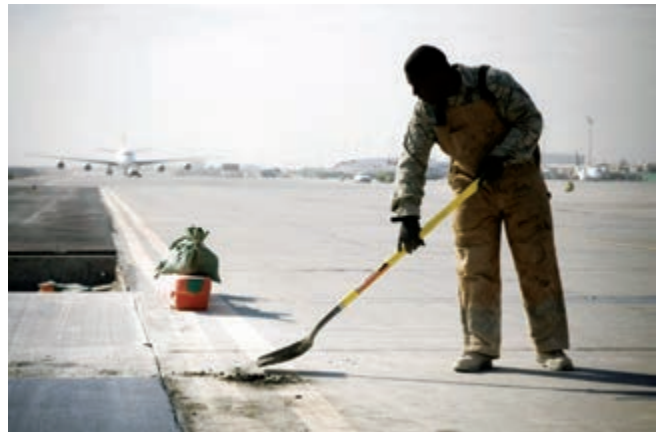
Working around construction machinery is a hazard on the airport runway. Image courtesy of pixabay.com
