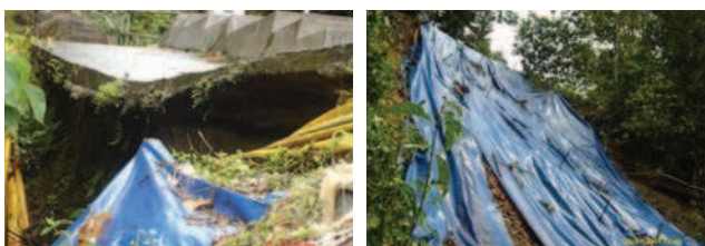
Figure 6: Sub-structure of track badly eroded
