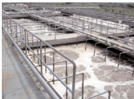
Figure 6 : MMF and Secondary Clarifier
