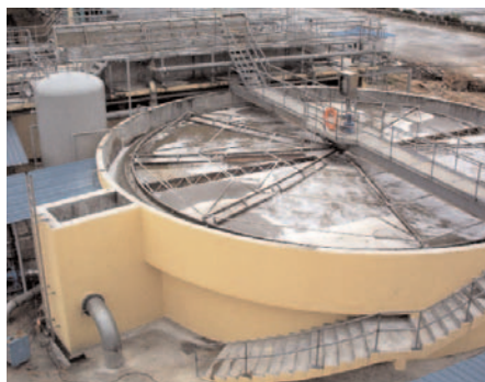
Figure 3 : Dissolved Air Flotation Clarifier
