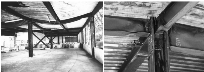
Figure 8: Ductile failure of steel structure due to fire (Bailey et al. [12], 1999; Allam, Burgess and Plank, 1999 [13]).
