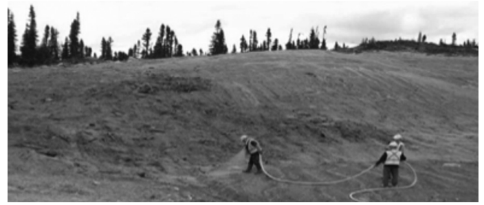
Figure 9: Hydromulching product sprayed on to soil to cover open slope area to be produced in UKM
