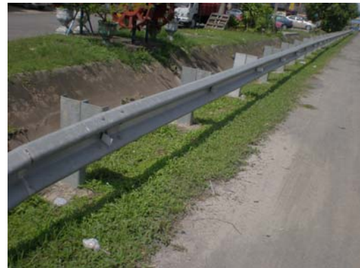
Fig. 1. Typical steel roadside safety barrier
