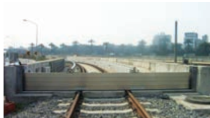
Flood barrier for rail tracks
