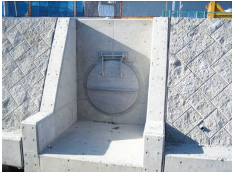
Flap gate for drain outlet
