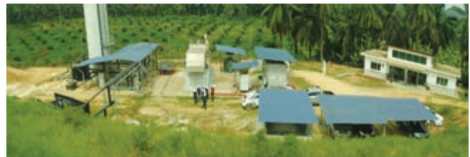
Sawira biogas power plant 1.0 MW (grid connection)
