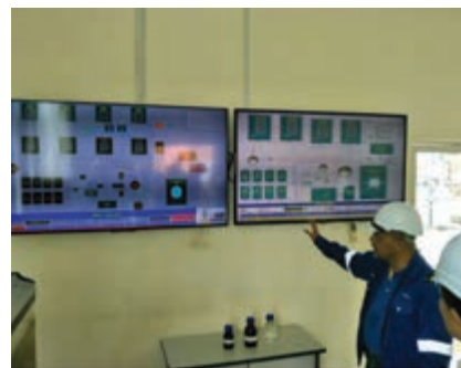
The SCADA system to monitor the leachate treatment processes
