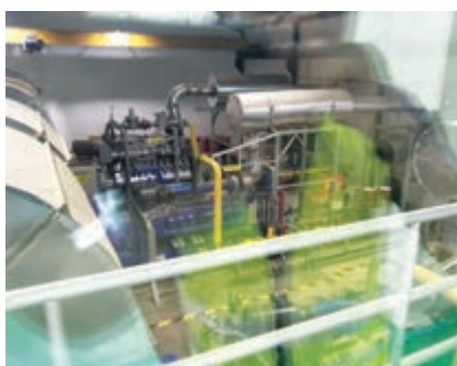
The gas engine units
