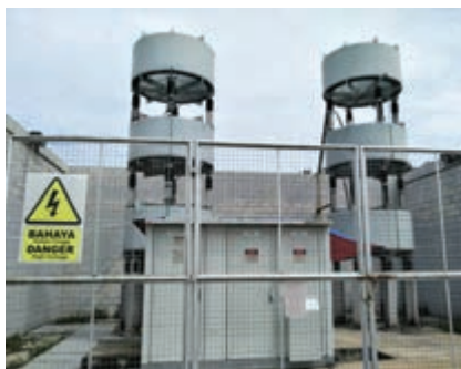
Interconnection to the Grid
