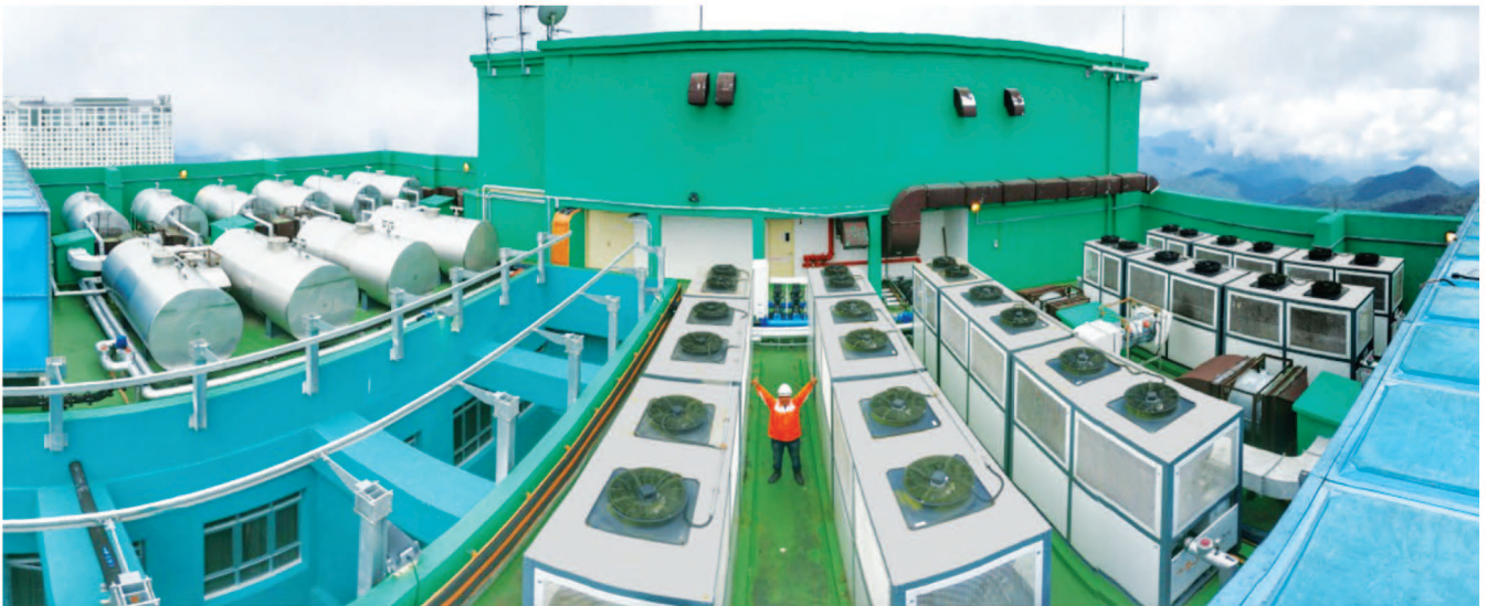
Intrix Heat Pump installation at First World Hotel in Genting
