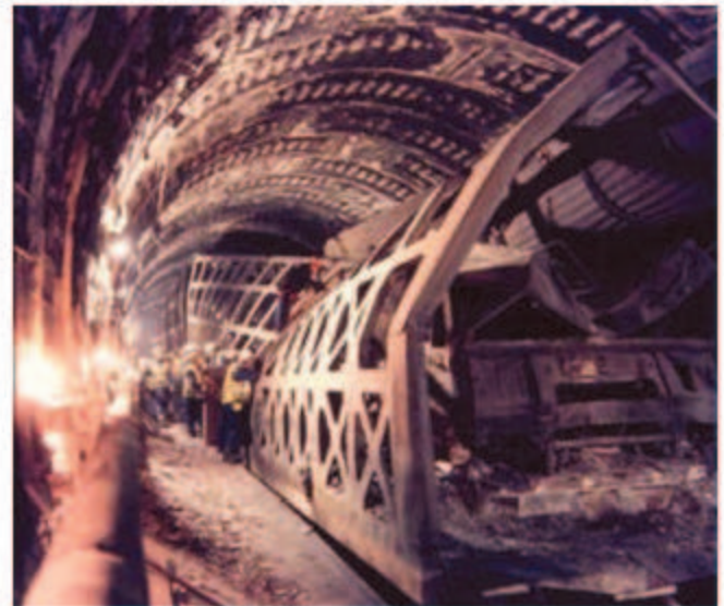
Channel Tunnel fire damage – ART (picture from subways.net)
