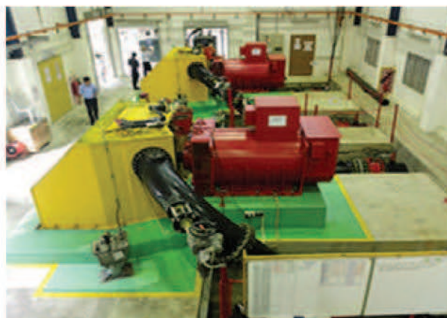
3 Turbines in Power Station
