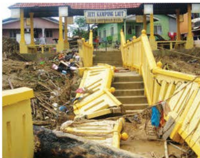
Part of Kampung Laut jetty in Kelantan collapsed when flood hit the state in 2014
