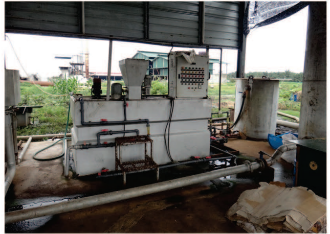
Photo 3: Multi disc screw dewatering press
