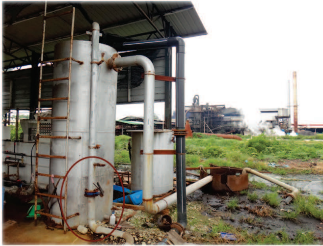
Photo 1: Balancing tank – Inlet and overflow
