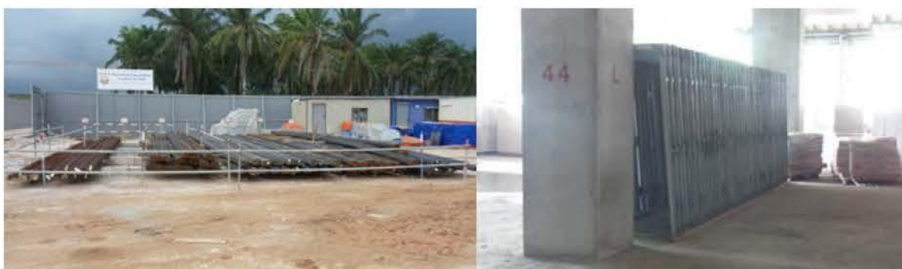
Door frames are stacked to prevent distortion and damage at Sunway Velocity Phase 2 Project
