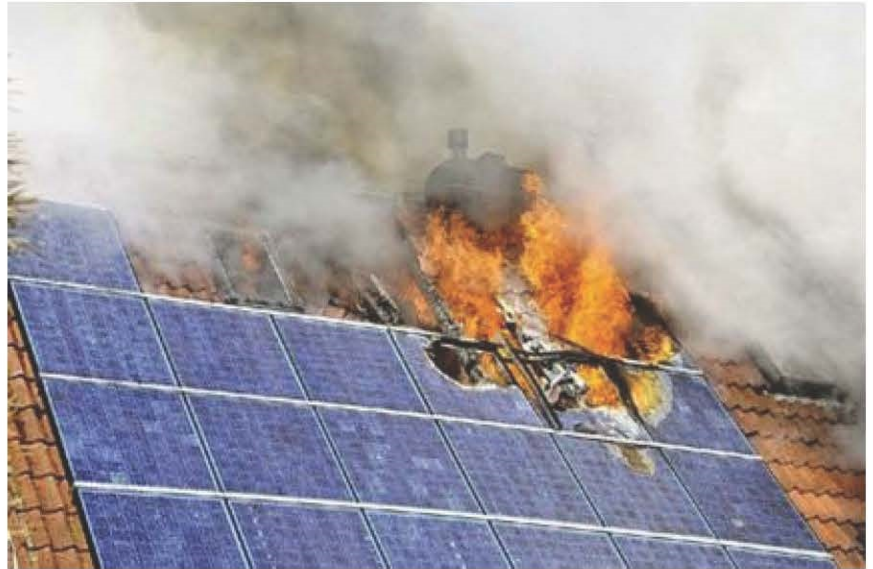
Roof Mounted Solar PV Fire (Source: solarexpert.wordpress.com)
