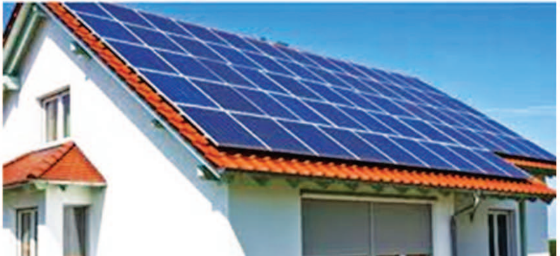
Domestic Roof Mounted Solar PV System (Source: pv-magazine)
