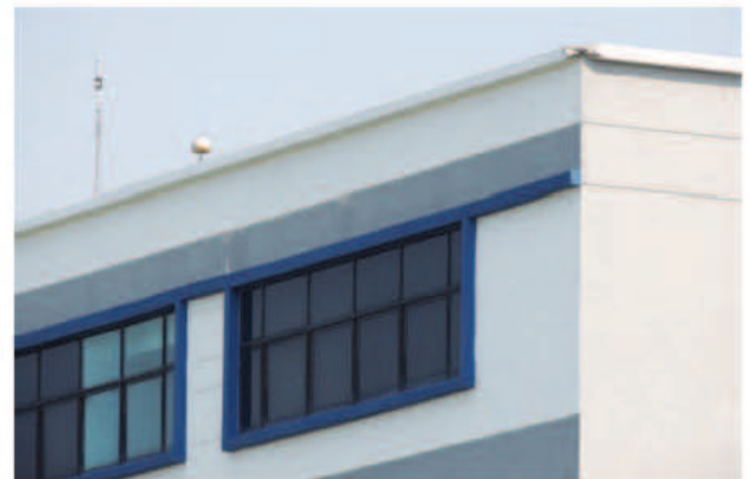
Figure 11: The same college building displaying a bypass after lightning struck a corner of the roof
