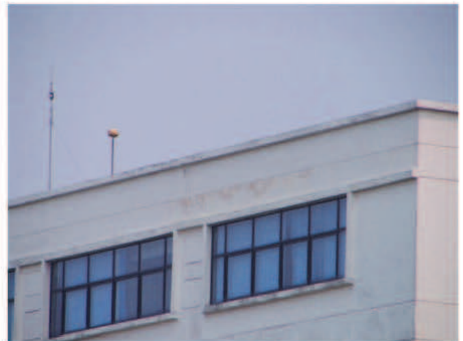
Figure 10: A college building installed with the ESE and CV air terminals before lightning struck
