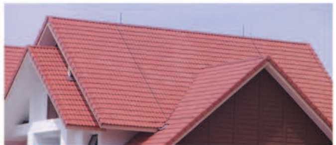
Figure 5: Incorrectly positioned conventional air terminal on a house
