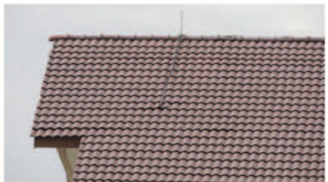
Figure 6: Incorrectly positioned conventional air terminal on a school
