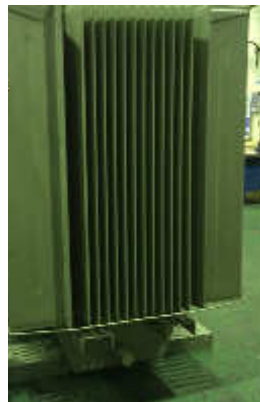
Transformers are ready for testing
