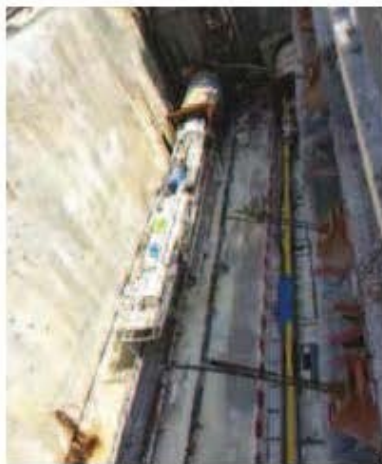
View of the assembly of the Tunnel Boring Machine (TBM) from above
