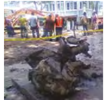
Damage at the site
