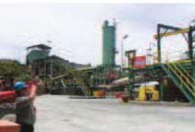
Part of the processing plant site showing the crusher, conveyor and milling sections
