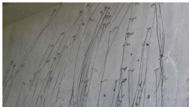
Figure 2: Crack monitoring of high strength ductile concrete
