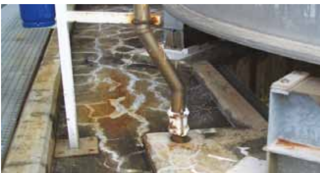
Figure 6: Widespread structural cracks
