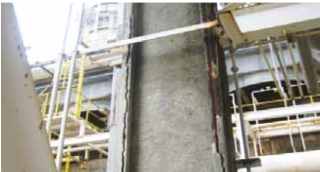
Figure 4: Structural cracks in concrete fireproofing
