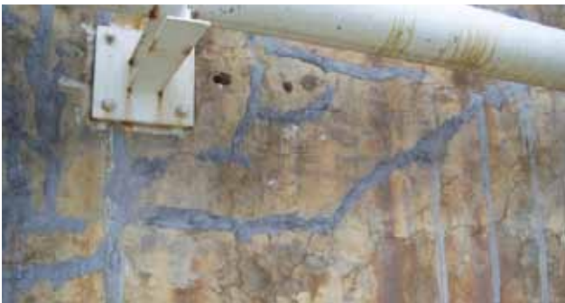
Figure 5: Structural cracks due to vibration
