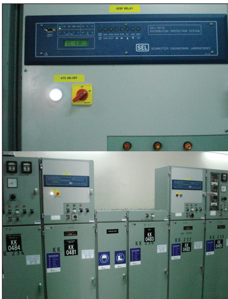
Above: The ATS indication light is on, showing that it is in operation. Below: ATS installation in SSU SUK Negeri Perak, Ipoh.
