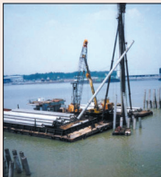
Railway Link Connecting Existing Railway Line to West Port, Pulau Indah, Klang, Selangor
