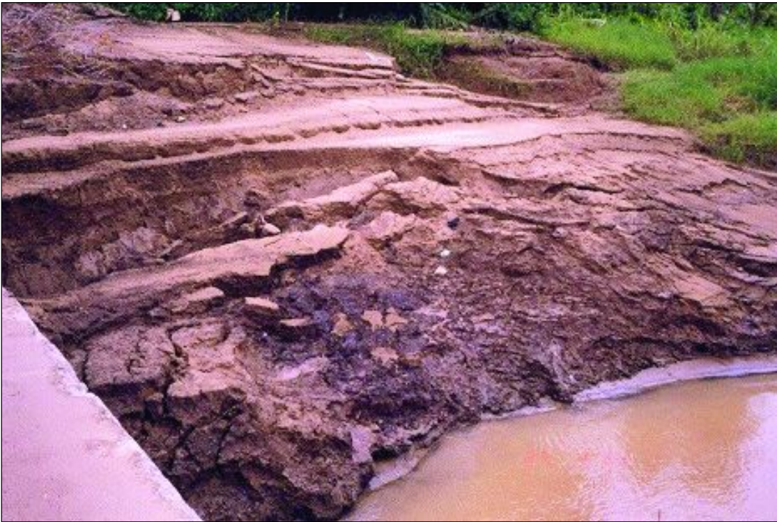
Figure 11: Riverbank instability, Sarawak
