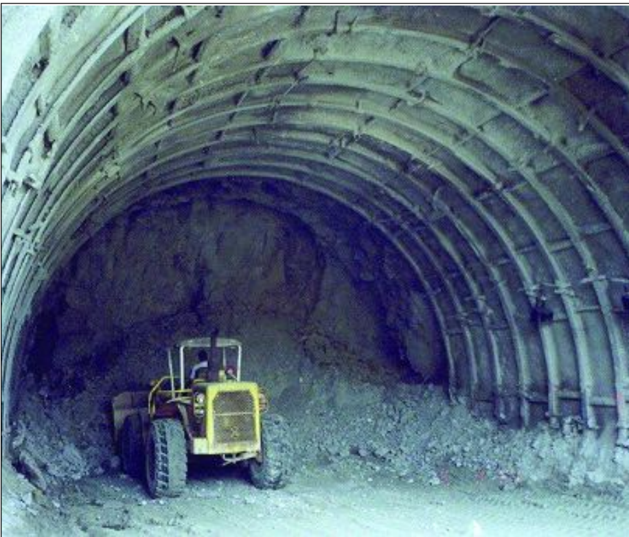
Figures 10a and 10b: Highly fractured granite and steel sets support, diversion tunnel, Sg. Selangor dam
