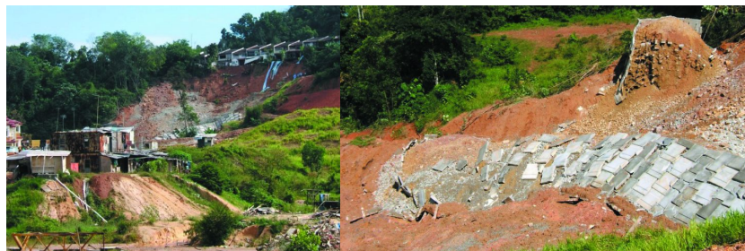
Collapse of reinforced soil wall at Kampung Pasir on 31 May 2006
