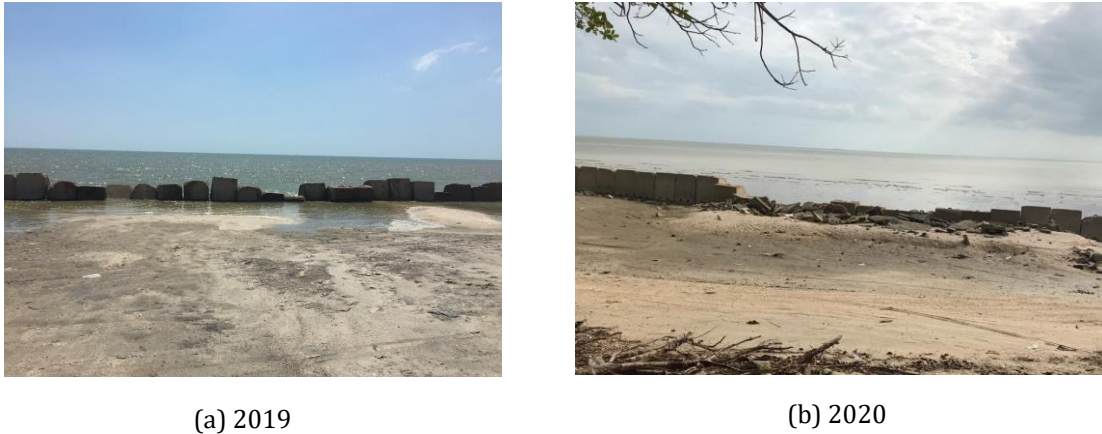
Figure 2. Condition of the Revetments (Labuan Blocks) Sungai Punggur in (a) 2019 and (b) 2020.
