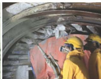
Application of fibre mortar shotcrete behind TBM (Picture courtesy of T. Matsumoto)
