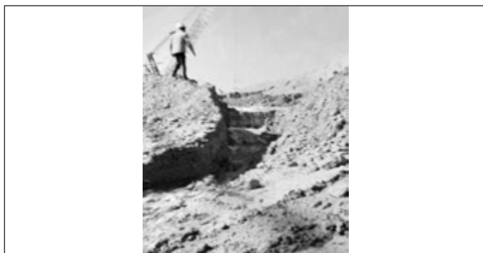
Figure 7: Dubai Dry Dock – rapid erosion of the downstream face of the bund.
