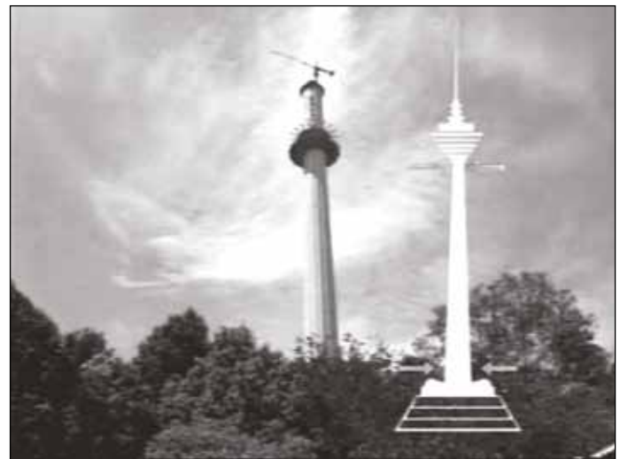
Picture 11.9: Using slip form, the concrete shaft of the KL Tower which stands at 360 metres, took only 4 months to build (Source: YTL)
