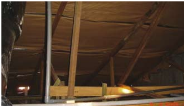
Figure 4: No proper bracketing (Source: http://www.azeetapipe.com )
