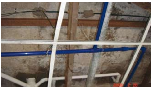
Figure 5: Thin wire used as pipe bracket (Source: http://www.azeetapipe.com )
