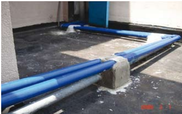
Figure 12: Exposed ABS pipe secured firmly with cement mortar (Source: http://www.azeetapipe.com )
