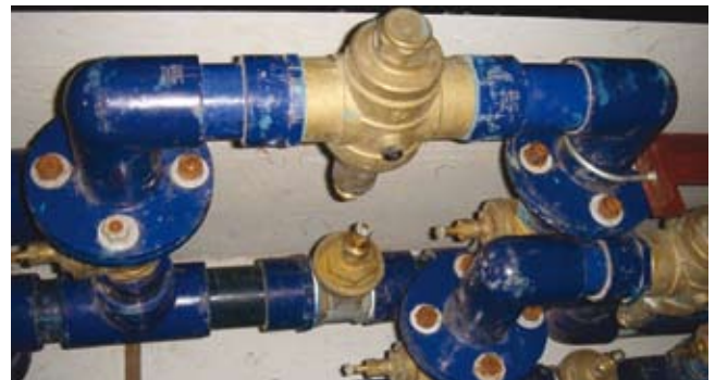
Figure 10: PRV installed without pressure gauges (Source: http://www.azeetapipe.com )
