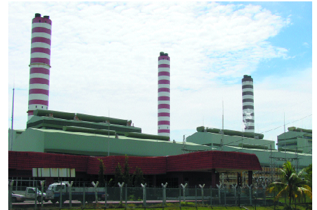
Sultan Salahuddin Abdul Aziz Power Station
