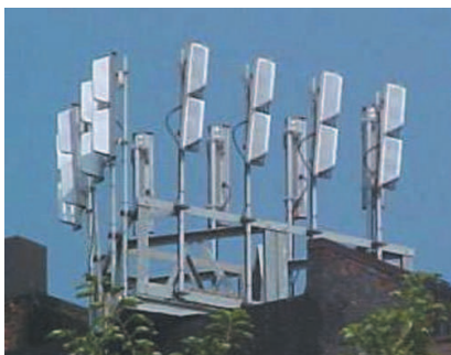
Figure 1: Base station antenna structure on a rooftop
