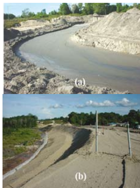
Figure 6: (a) Flow channel for material transport at the crest of the embankment and (b) construction of rock toe wrapped with geotextile
