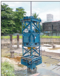
A 30-metric tonne hammer that can be used to test in excess of 2500 tonnes! Normally, PDA tests can be tested using the piling hammer used to drive the piles in the case of pre-cast concrete and steel piles. However, in situations where the piling hammer is not available, drop hammers such as this one will be deployed.
