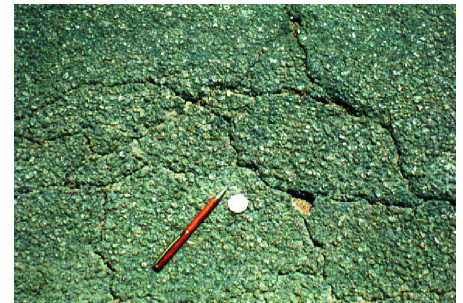
Figure 2a: Fatigue cracking
