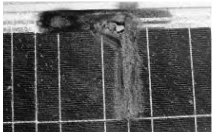
Figure 2: Damaged PV Module Aluminum Frame Caused by Lightning Stroke Attachment
