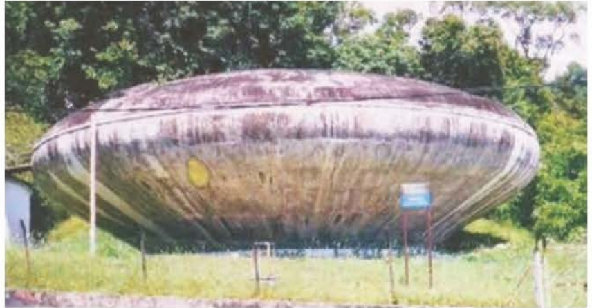
A 900,000-litre water tank
