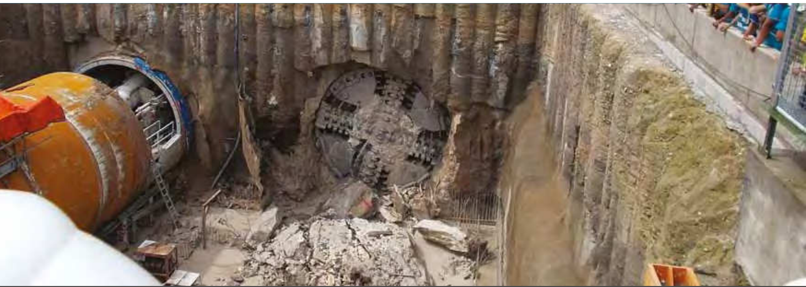
Photo 1: TBM breakthrough at KVMRT Maluri Station in April 2014 (Picture courtesy of Ir. CK Lee)
