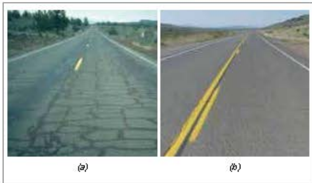
Figure 1: (a) before and (b) after using rubberised binder overlay after 16 years of performance [6]
