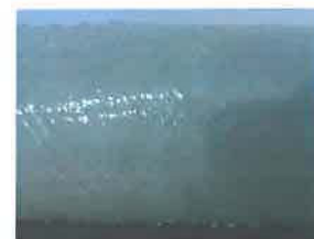
Weepage failure in composite pipe at high pressure
