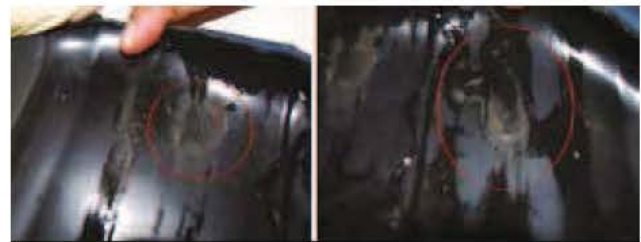
Figure 3: Burn mark at the insulation (Y-phase).
