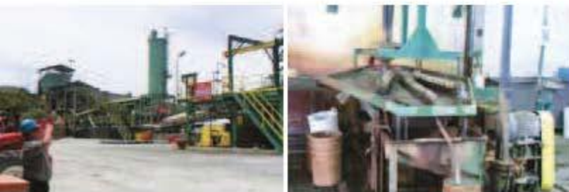
Part of the processing plant site showing the crusher, conveyor and milling sections The shaking table used to collect gold nuggets or coarse gold particles
