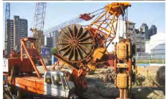
Figure 2: Slurry wall construction with horizontal and vertical site constraints, and modified slurry wall equipment
