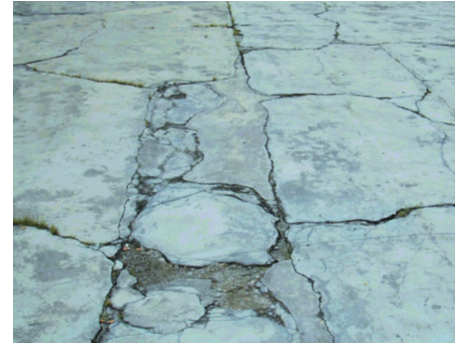
Figure 5: Cracks in walkways due to no proper construction joints
