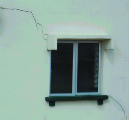
Figure 14: Structural cracks due to differential settlement
