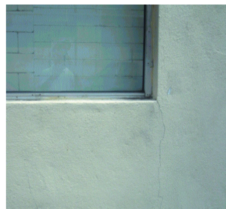
Figure 13: Common shrinkage cracks at window areas
