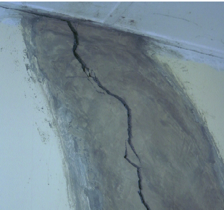
Figure 15: Cracks which are moving or progressing cannot be repaired with cementitious mortar
