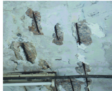
Figure 10: Corrosion of reinforcement can be a huge problem in marine structures
