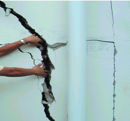
Figure 12: There is no need to evaluate this crack, its serious damage!
