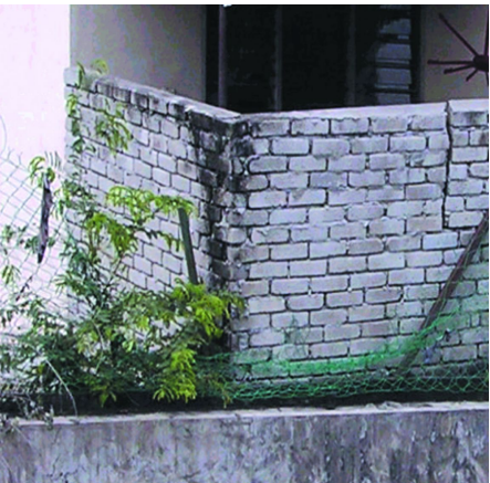
Figure 9: Cracking of brickwall extension because of differential settlement
