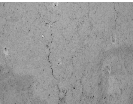
Figure 3: Plastic shrinkage cracks caused by rapid evaporation of water
