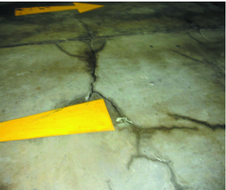
Figure 7: One of the most common places to find cracks is underground car parks
