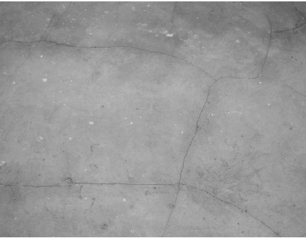
Figure 2: Typical shrinkage cracks in floor slabs
