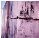
Structural crack on a water retaining structure
