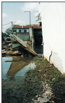
Collapse of a water retaining structure
