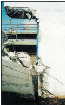
Collapse of an Aeration Tank
