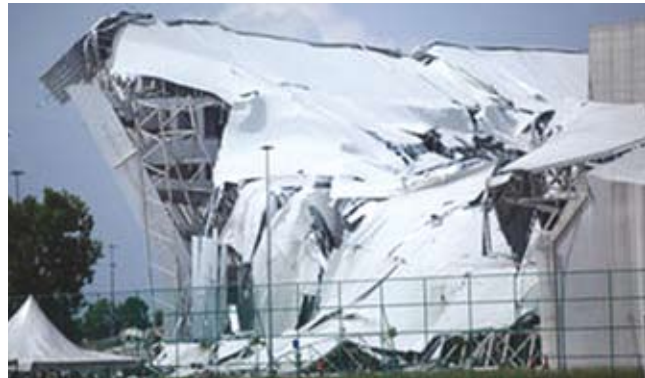
Figure 9: The damaged portion of the stadium - (Courtesy of NORDIN A. RASIP)
