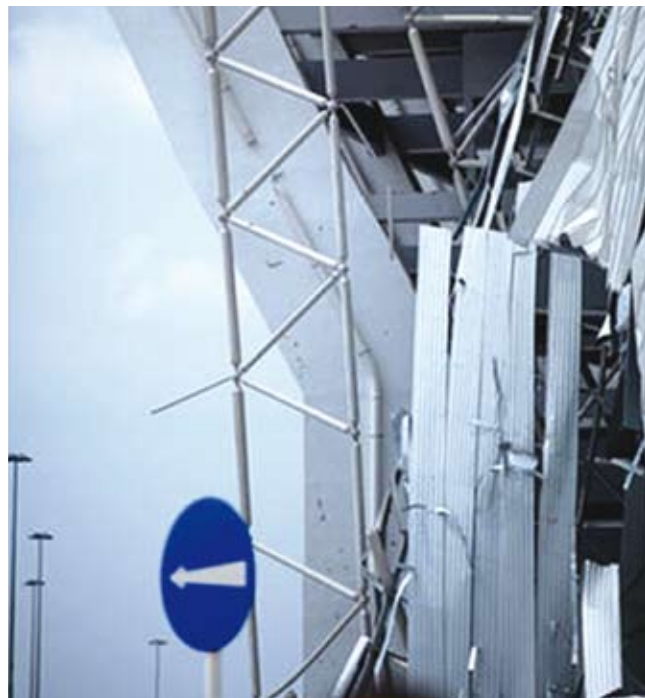
Figure 10: Part of the caved-in structure - (Courtesy of NORDIN A. RASIP)
