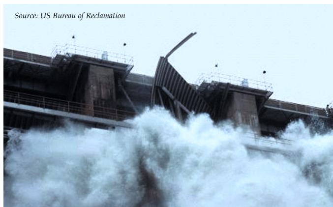
Failure of the spillway gate at Folsom Dam, USA (July 1995)
